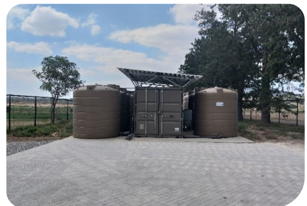
Mariendahl borehole and filtration system
