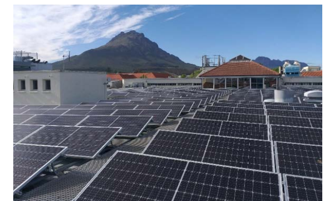
Photo: Solar photovoltaic installation on the roof of the Neelsie Student Centre.
