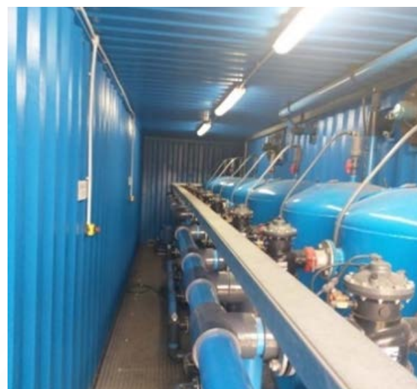
Photo: Inside the reverse osmosis plant at Bellville Park campus
