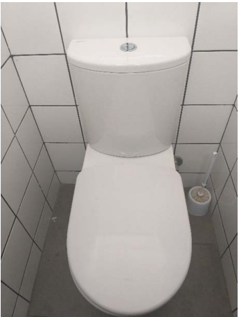
Photo: Water efficient toilets
