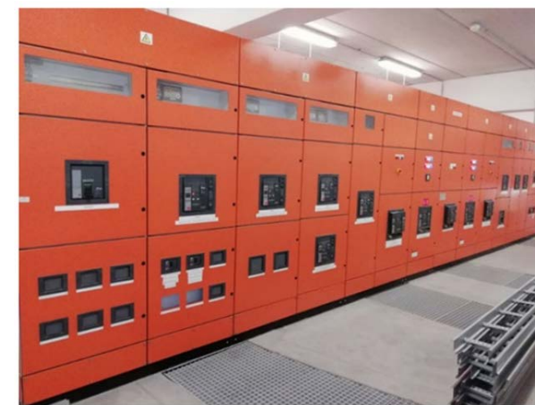
Photo: Energy metering
