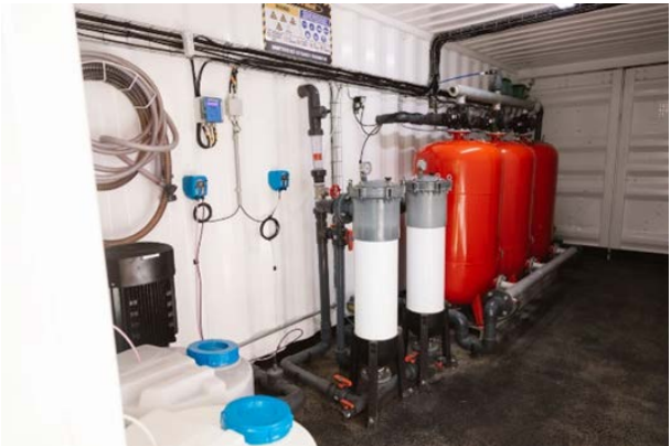
Photo: Grey water filtration plant
