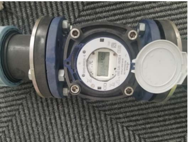
Photo: Water meter
