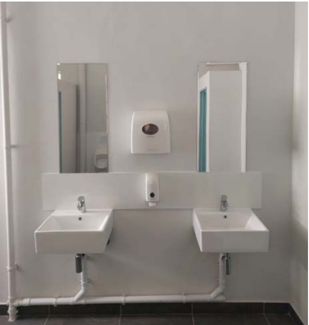
Photo: Water efficient taps
