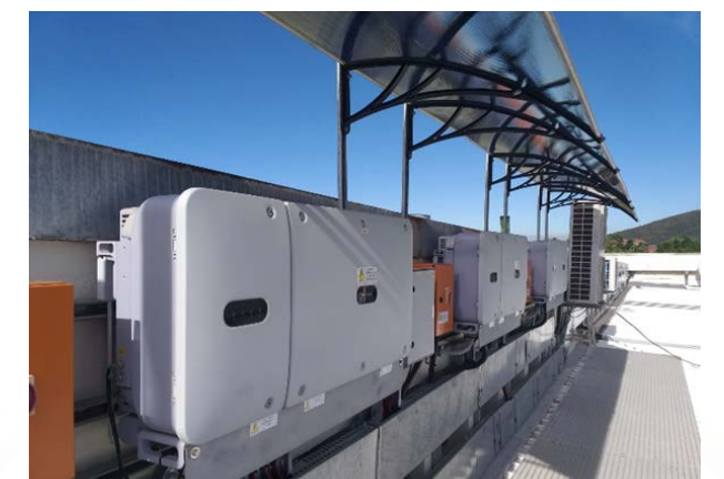
Photo: Inverters at Neelsie Solar Photovoltaic installation
