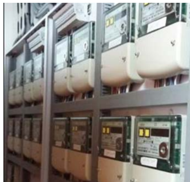
Photo: Energy meters
